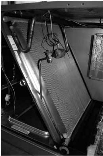
Evaporator Coil/Filter Access
