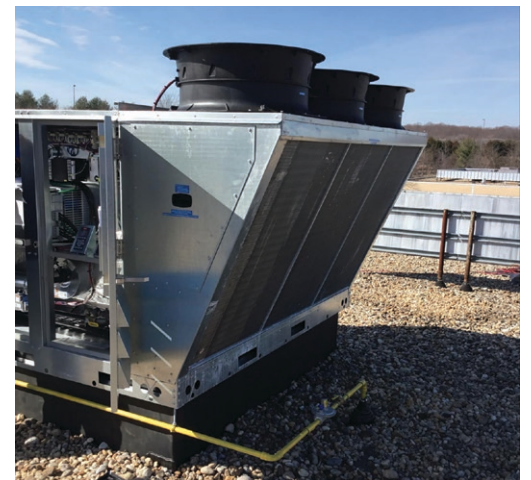
Installed DOAS unit at the Laboratory
