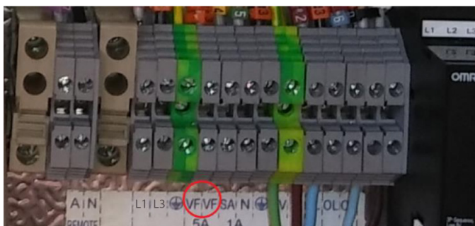
Picture of heat pump terminal strip.
