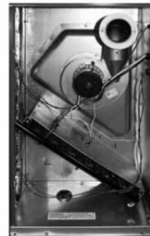
Heating Compartment Access
