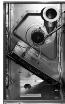
Heating Compartment Access
