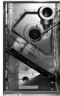
Heating Compartment Access
