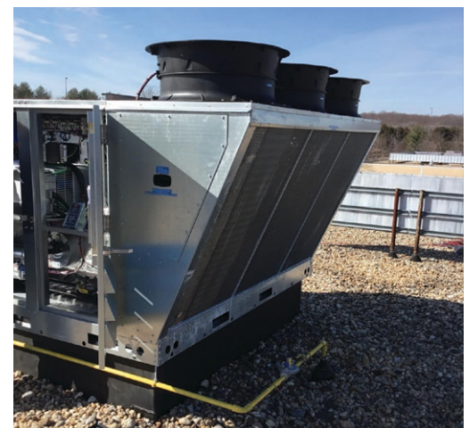
Installed DOAS unit at the Laboratory
