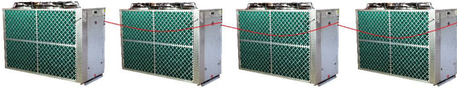
1st Heat Pump / Primary 2nd Heat Pump Secondary 1 3rd Heat Pump Secondary 2 4th Heat Pump Secondary 3
