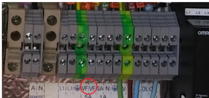
Picture of heat pump terminal strip.
